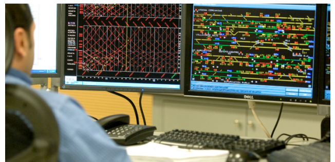
Traffic Management at central control room
