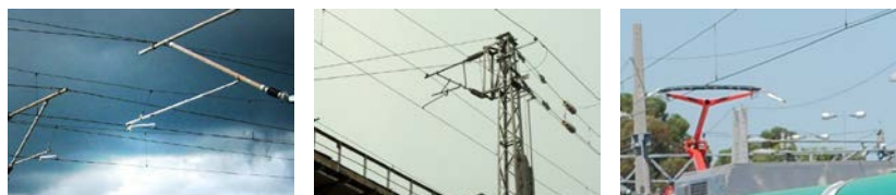
1) Wire of Catenary incl. Overhead wiring
